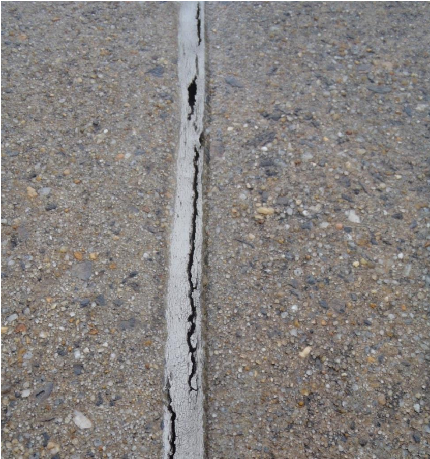
Cohesive Failure/Aged & Weathered
