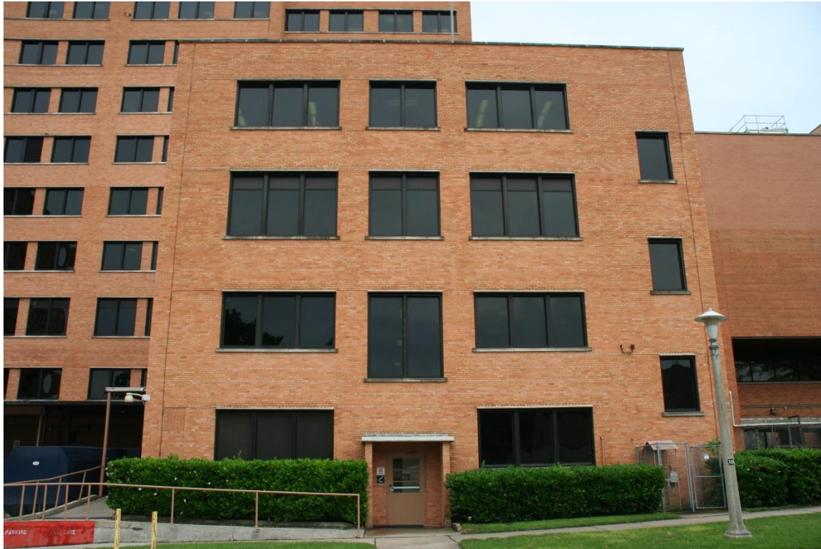
No Expansion Joints
