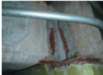
Figure 5 Rebar corrosion and failed repair
