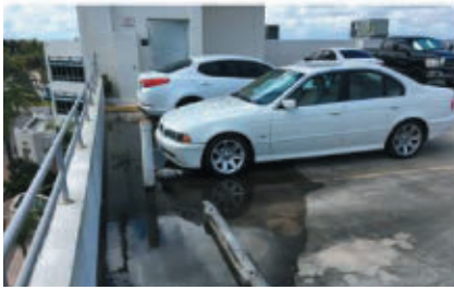
Figure 3 Ponding and concrete spall
