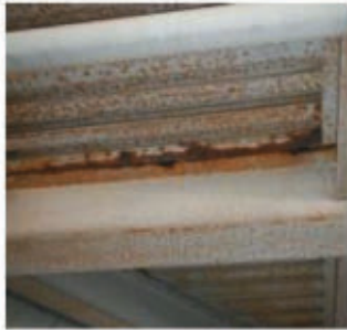
Figure 9 Rusting structural steel and metal deck
