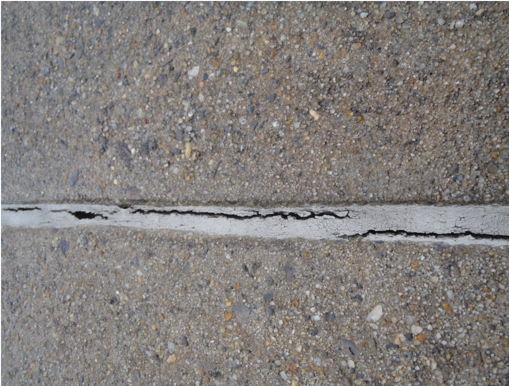
Cohesive Failure/Aged & Weathered
