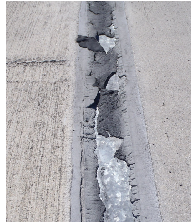
Expansion Joint Failure
