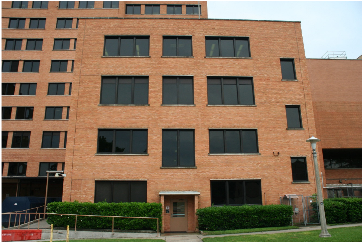
No Expansion Joints
