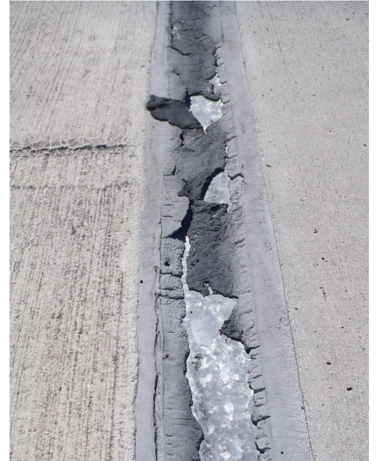
Expansion Joint Failure
