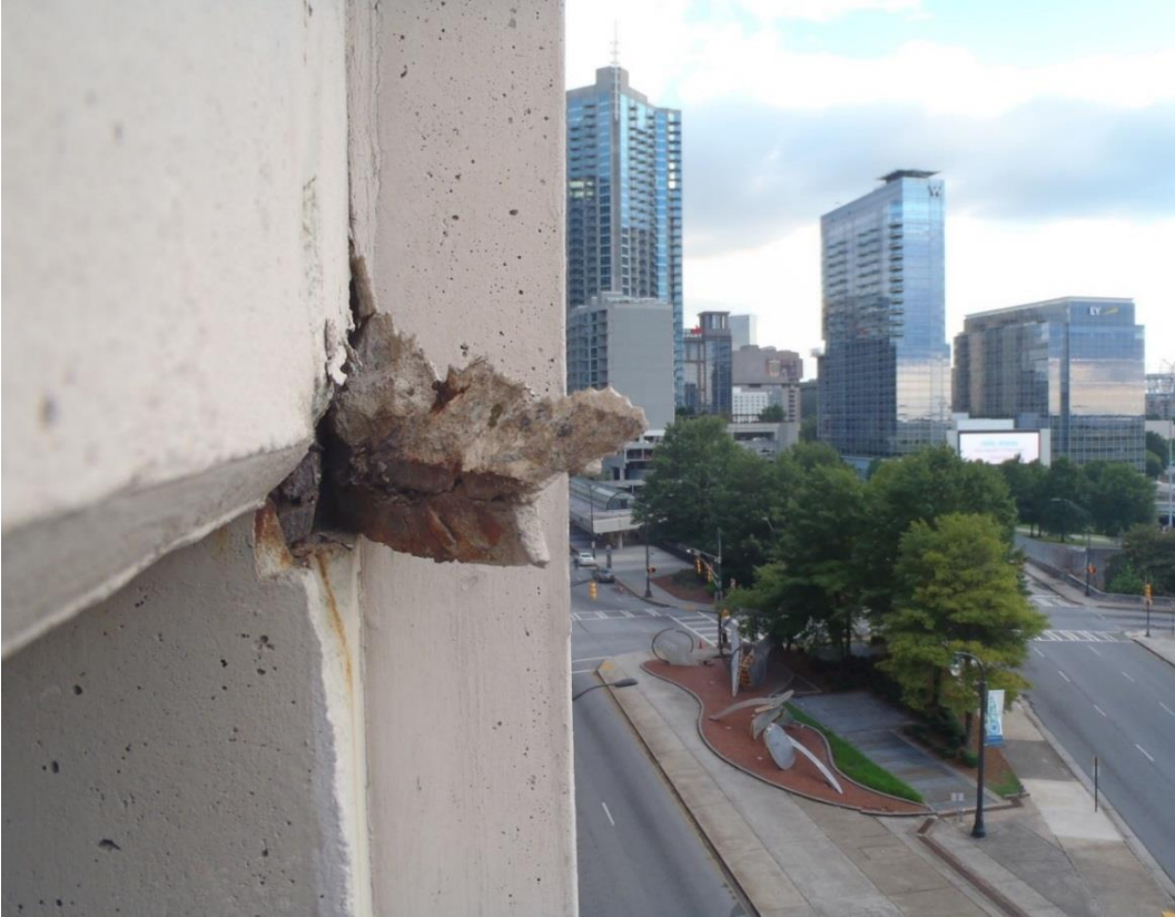
Spall Over Sidewalk
