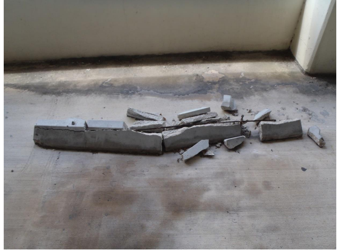
Broken Wheel Stop
