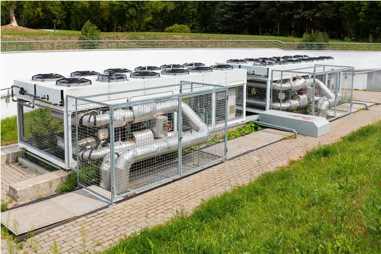
Ground Supported Equipment
