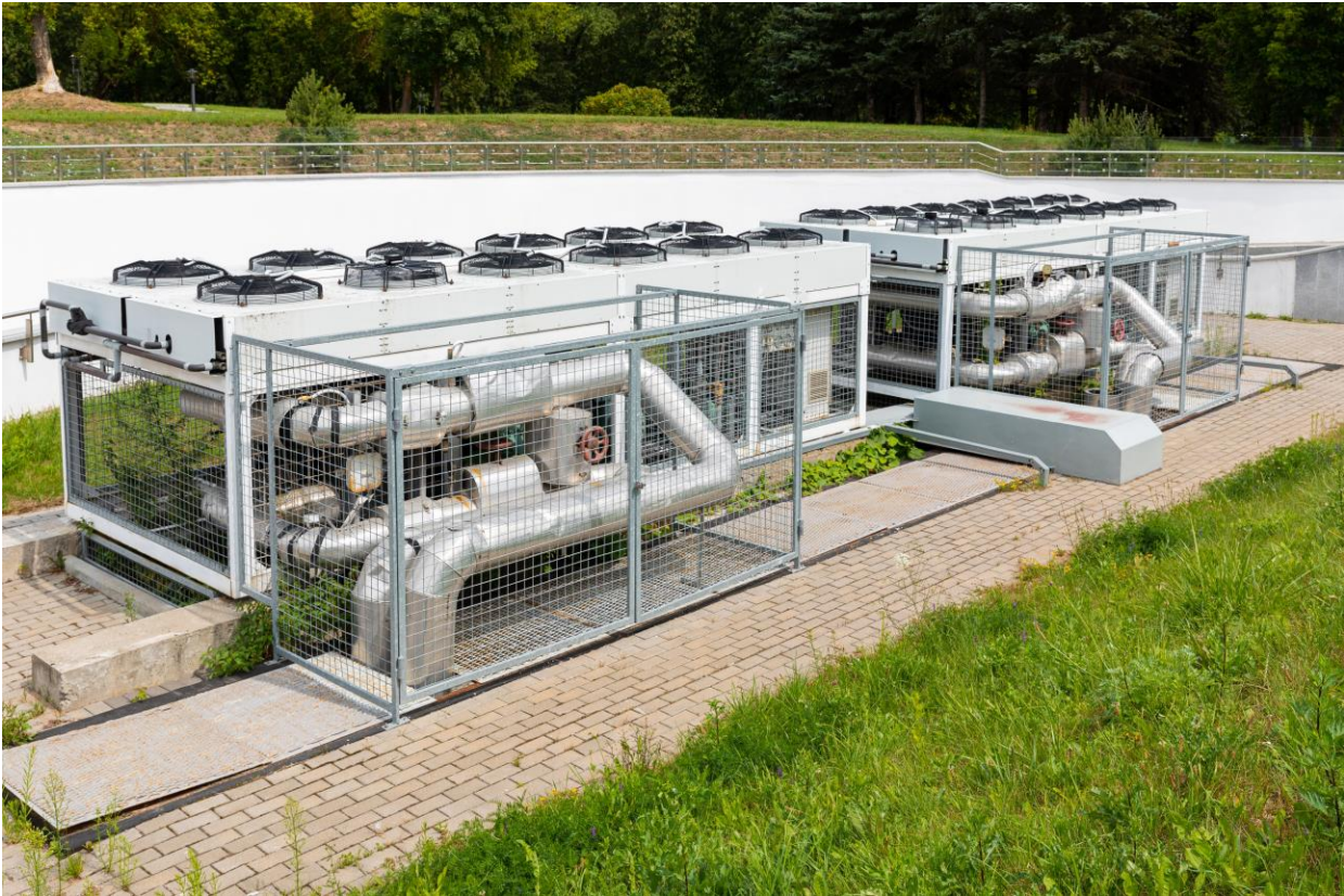
Ground Supported Equipment
