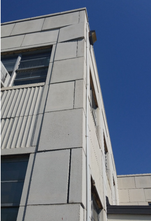
Level D: Loose Stone Panels
