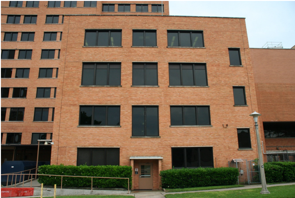
No Expansion Joints
