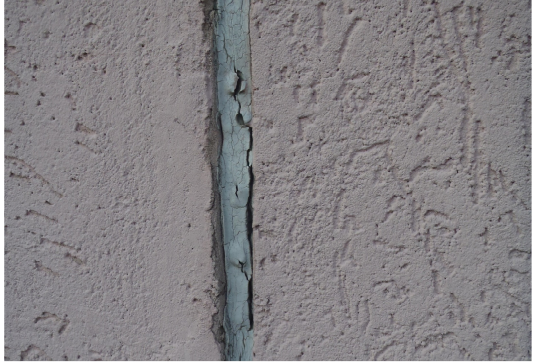
Level B: Failed Sealant
