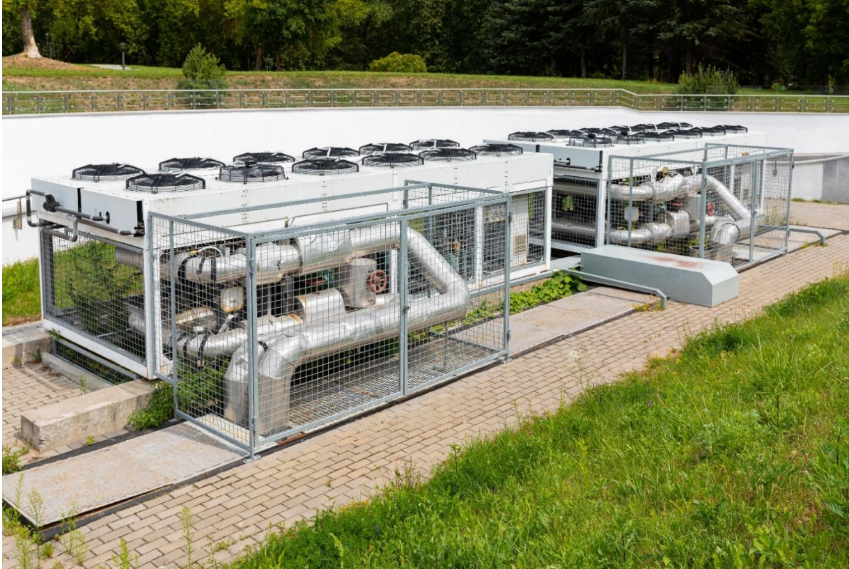
Ground Supported Equipment
