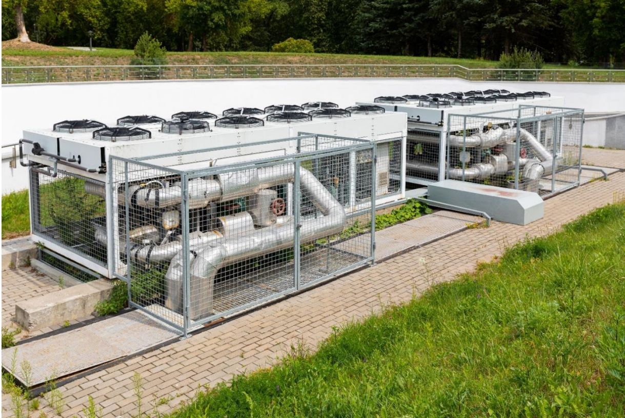
Ground Supported Equipment
