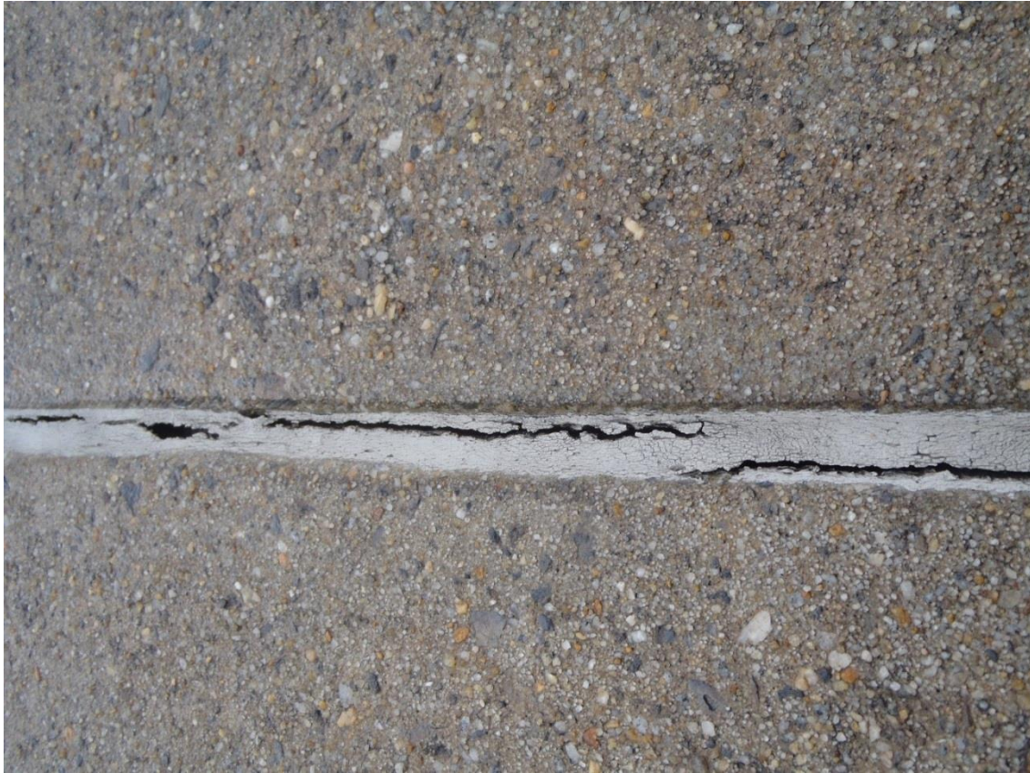
Cohesive Failure/Aged & Weathered
