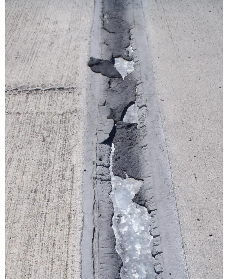
Expansion Joint Failure
