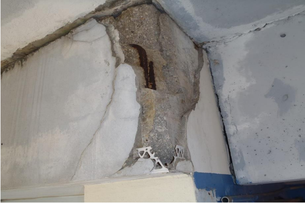
Rust Expansion & Spalling
