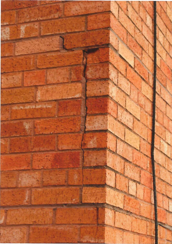
Cracked corner brick resulting from lack of expansion joints in brick veneer
