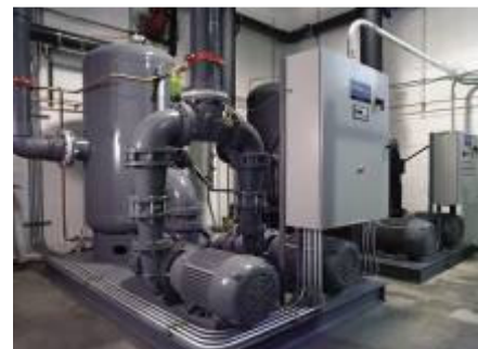
Example Pumping Station
